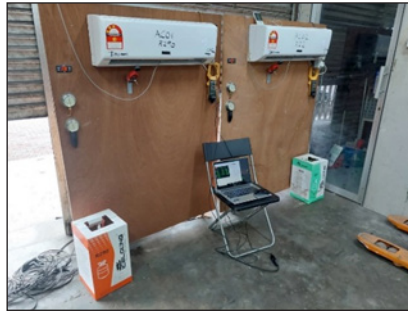
Figure 3. Complete indoor evaporator blower setup with measurement gadget
